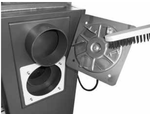
Sample cleaning of impeller and checking uprightness of vane on extract ventilator
