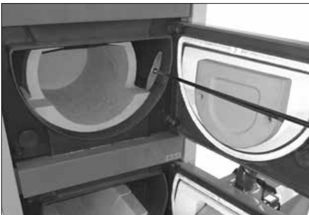
Open middle space of the boiler with a roof and example of ash removal with a poker
