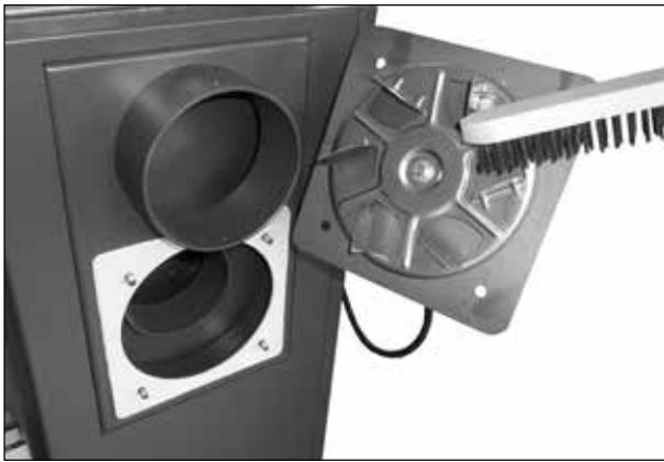
Sample cleaning of impeller and checking uprightness of vane on extract ventilator
