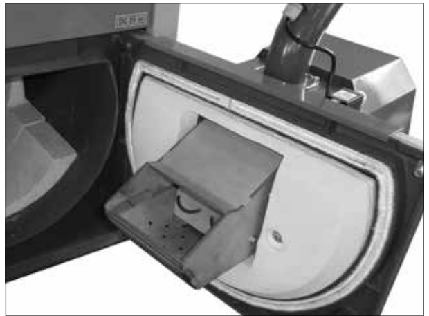
Open bottom door of the boiler during cleaning of the combustion chamber of the burner ATMOS A25
