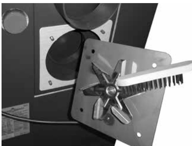
Sample of impeller cleaning and checking of vane on extract ventilator
