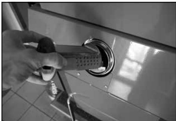
Example of inserting the ignition chamber into the boiler
