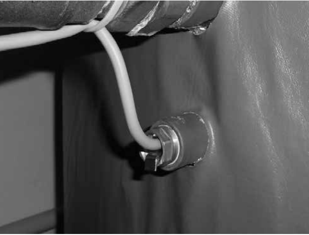
Fig. 13 – View of the water temperature sensor in the pocket of the accumulation tank (TV and TS)
