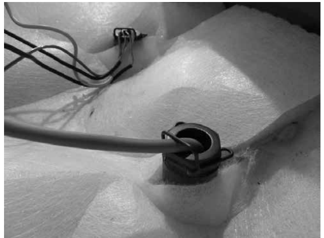
Fig. 16 – View of the water temperature sensor TK in the boiler pocket, DxxP, Pxx types
