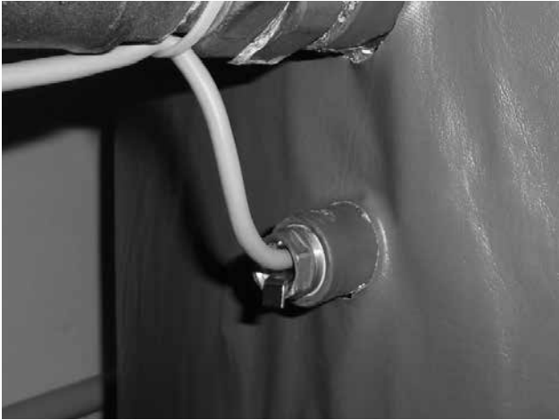
Fig. 13 – View of the water temperature sensor in the pocket of the accumulation tank (TV and TS)
